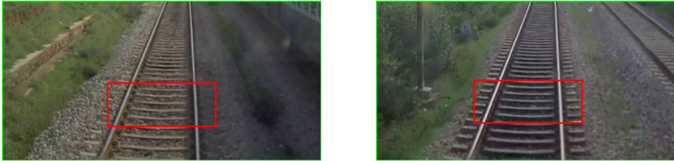
Figure 10: Normal Ballast (Left) Versus Loose Ballast (Right)
